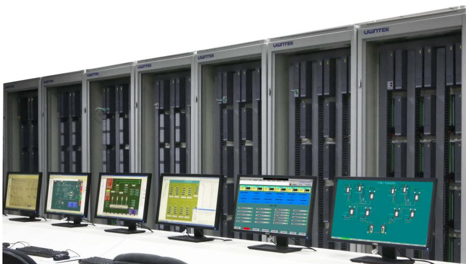
UW500 Distributed Control System Control Stations
